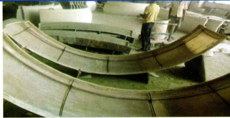
Balcony mold in FRP
